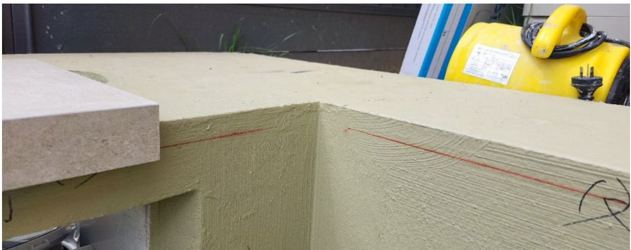
Image 3 - Appropriately designed and prepared substrate (including waterproofing system) ready for tile application.
